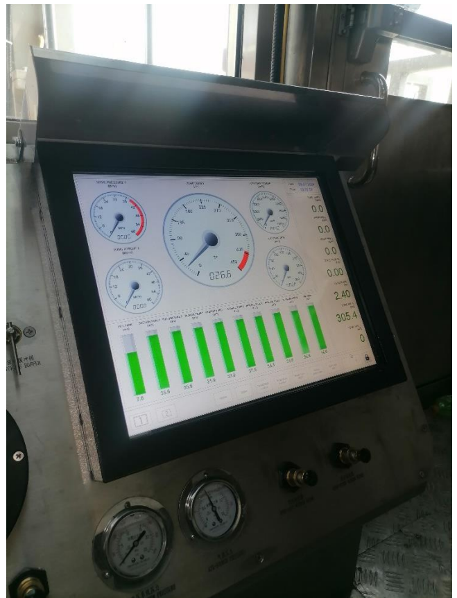
Figure 2. The MV-150(S) installation example in the driller's cabin
